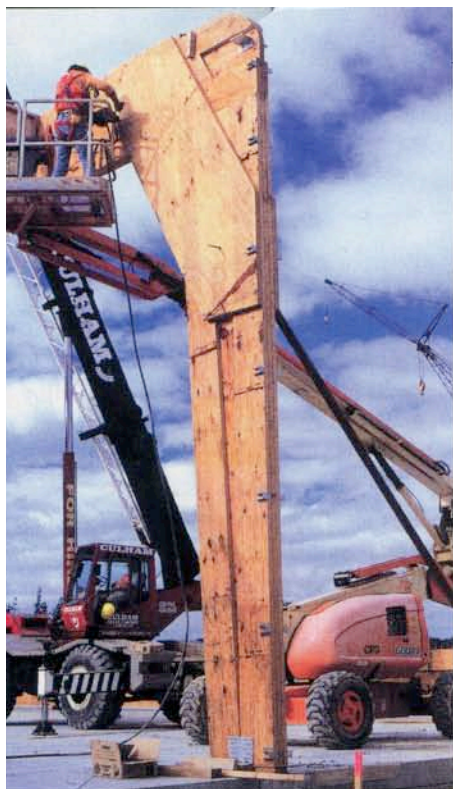
Mainzeal Construction used 620m 3 of LVL, 50m 3 of plywood timber and 15m 3 of sawn and dressed timber to build the structural frame of the main building.
